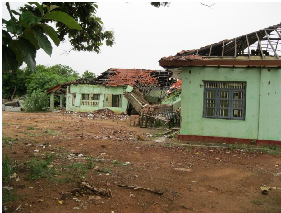
Another photo of the damaged hospital
