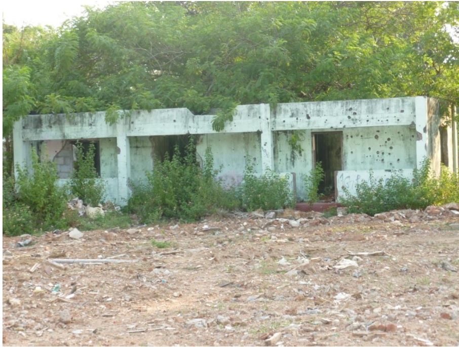
Damaged Mortuary of PTK hospital in August 2013
