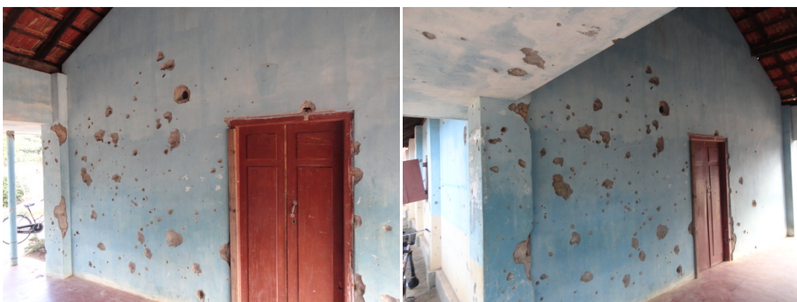
Photos 13&14: An office by the entrance of Iranaippalai GTM School with scars of war
