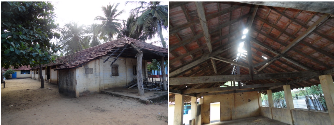
Photos 17&18: A damaged building that can be repaired at Iranaippalai GTM School
