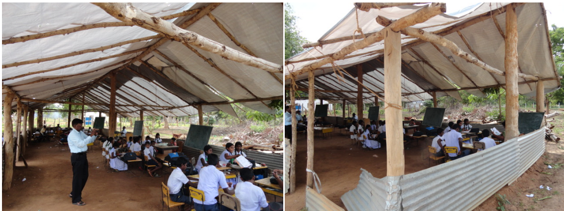
Photos 7&8: The damaged temporary shelter in Photo 6 is used as classrooms - Nov 2013
