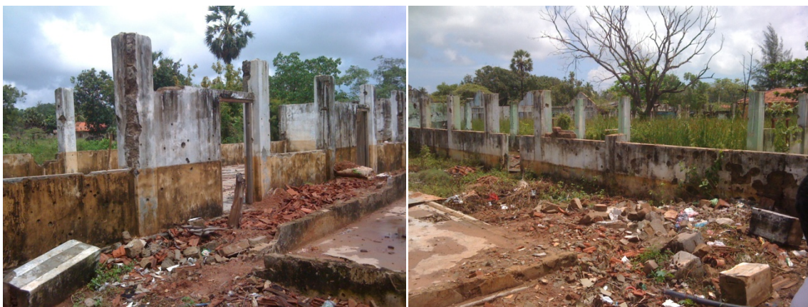
Photos 25&26: Damaged buildings of Sri Subramaniam Vidyalayam
